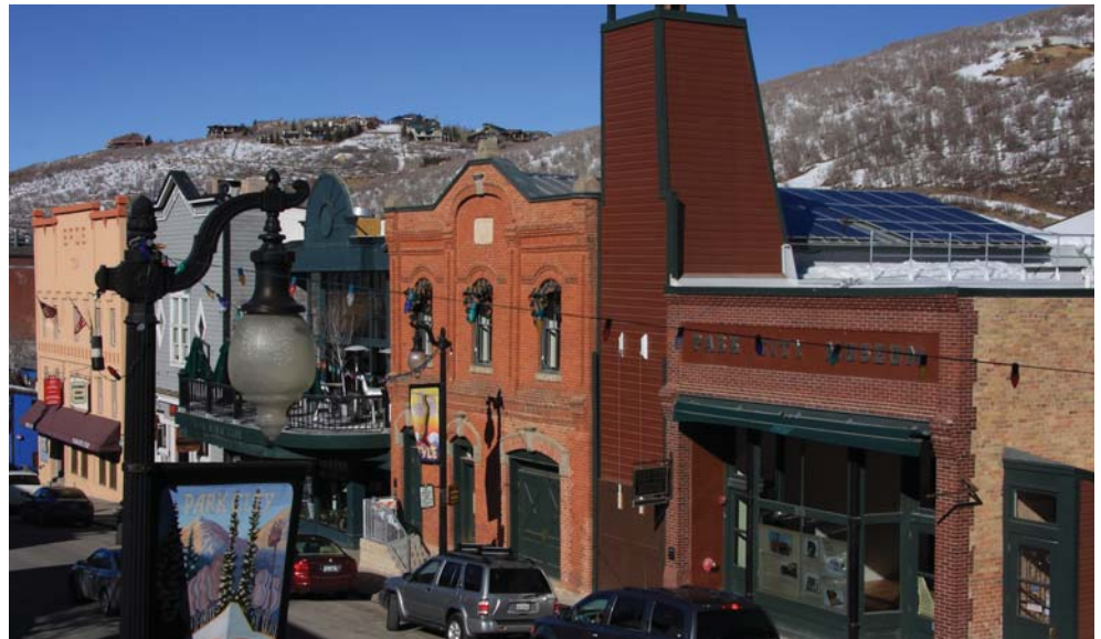
Layton's Interior Construction Specialists gave the Park City Museum a 5,400-square-foot expansion and facelift, bringing new use to an historic part of downtown.
